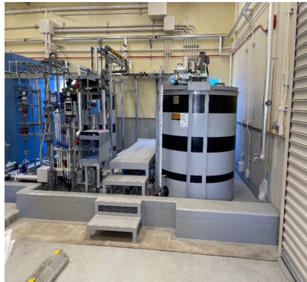
Figure 2: Sodium Hypochlorite & Fluoride Tanks
